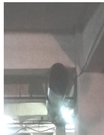
Gambar 24. Ventilasi mekanik Parkir Basement MBK
